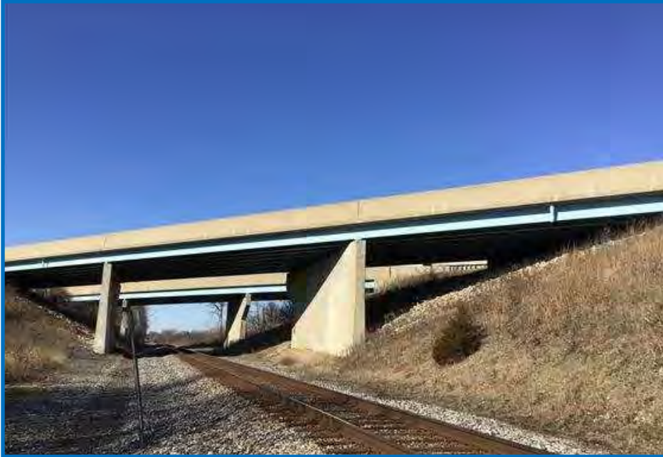
Photo 5— View of EB and WB I-70 Bridges over the Norfolk Southern Railroad Facing North (01/08/2020).
