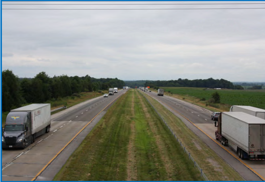
Photo 1— View along I-70 in Wayne County. Travel lanes will be added to the median (07/26/2022).
